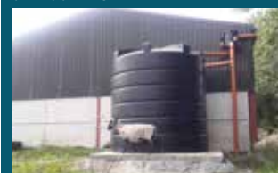
Fig. 3 Rainwater Harvesting System on Roo River
